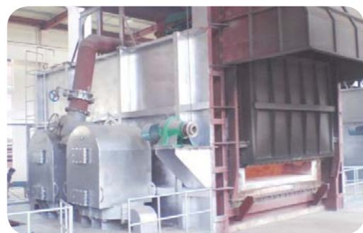
熔铝炉 Aluminium melting furnace
