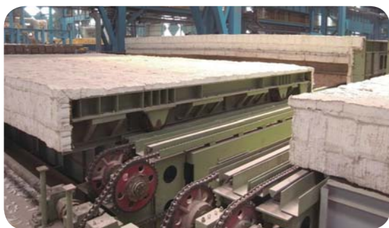
大型钢坯保温炉 Large billet holding furnace
