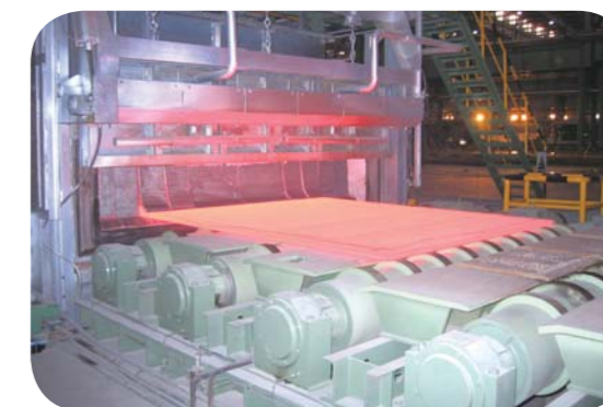
辊底式热处理炉 Roller hearth type heat treatment furnace
